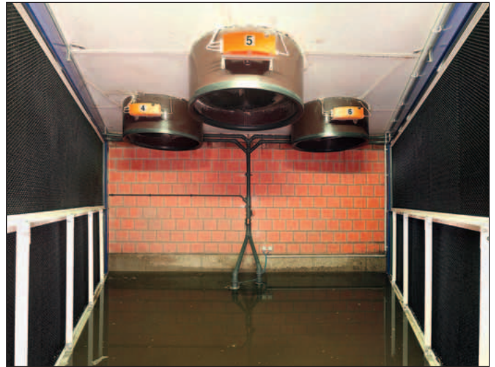
Back view of the filter – exhaust air chimneys suck the house air through the filter
