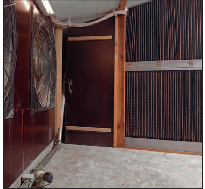
Rear side of the filter, ventilators suck the air through the filter wall
