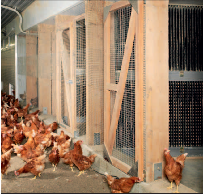
Using a StuffNix dust filter in an aviary house
