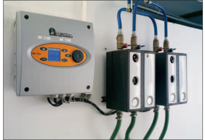
Climate computer MC 235 for control of the entire house climate; three-way control of warm-water heating system
