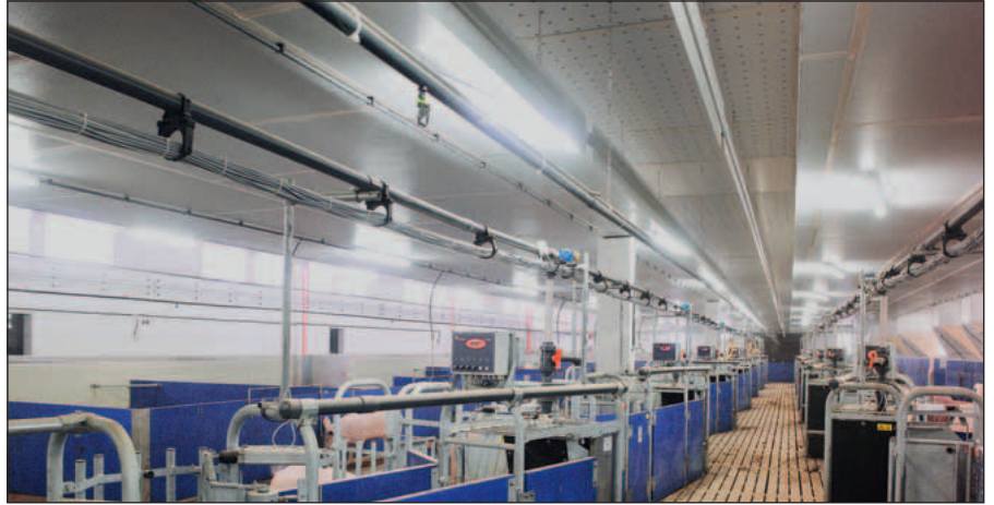
Fresh air supply over spray-cooling channel in the waiting area
